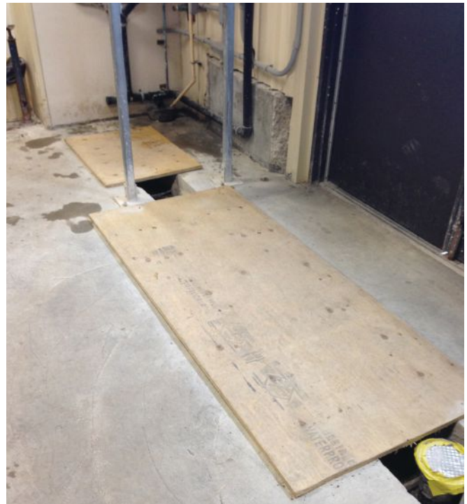
The floor drain was relocated to make room for the new RPU panel.
