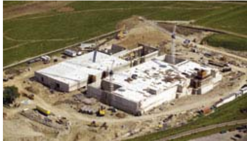
Precast concrete Airport Road Reservoir and Pumping Station will help meet region's burgeoning water needs. (Photo courtesy of Kenaidan Contracting Ltd.)
