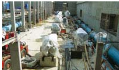
Team was challenged by large suction headers and multi-zone discharge headers in large pumping station. (Photo courtesy of Peel, Water & Wastewater Treatment)
