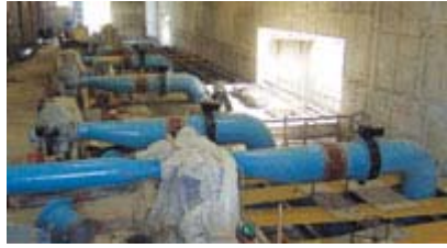
Massive pipes and pumps will control water flow from the 9.2-million-gallon, four-cell, underground reservoir.
